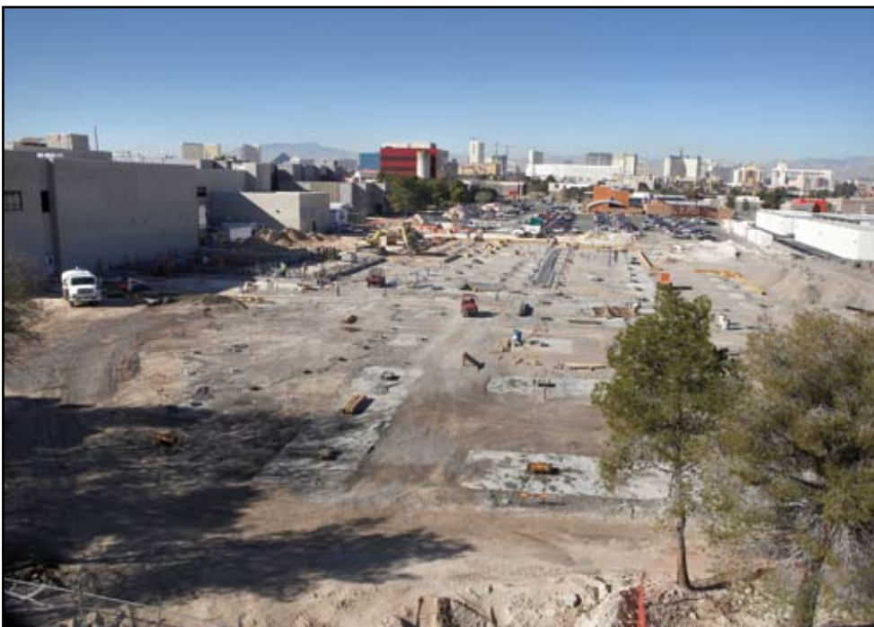
Construction continues on the Science, Engineering and Technology, slated for completion in 2008.
